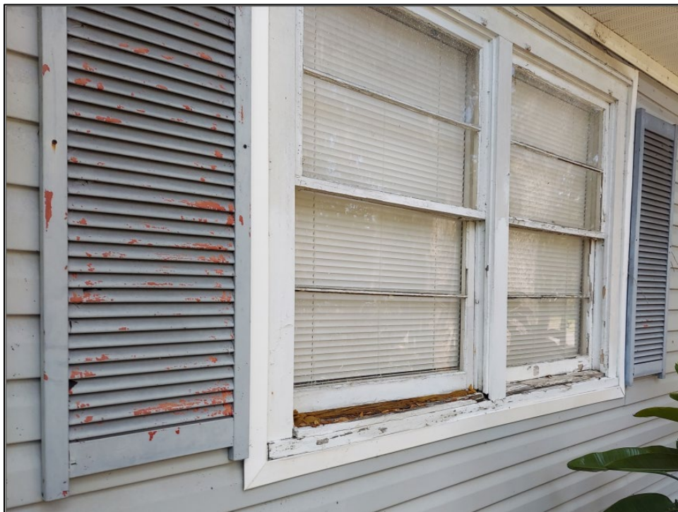
Figure 2: Applicant photograph of historic double-hung two-over-two sash window at façade. Deteriorated glazing, failing paint, and rotting at sills are visible.
