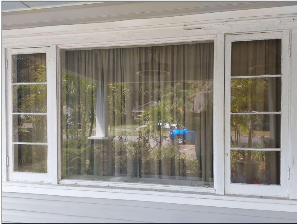
Figure 1: Applicant photograph of picture window at subject property's façade. Failing paint indicating possible rot or termite damage is visible at the casing above the window.
